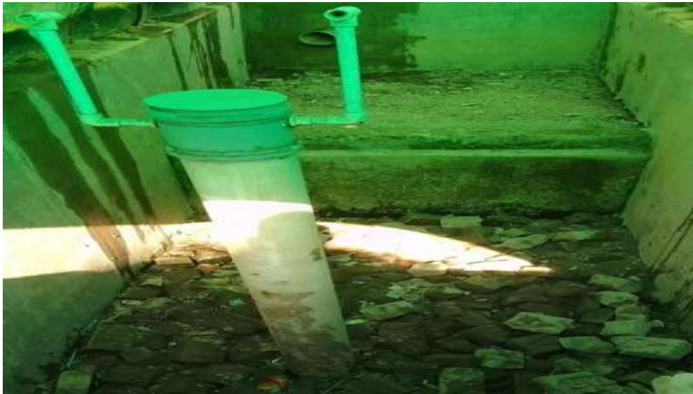
C11: Rainwater Harvesting System
