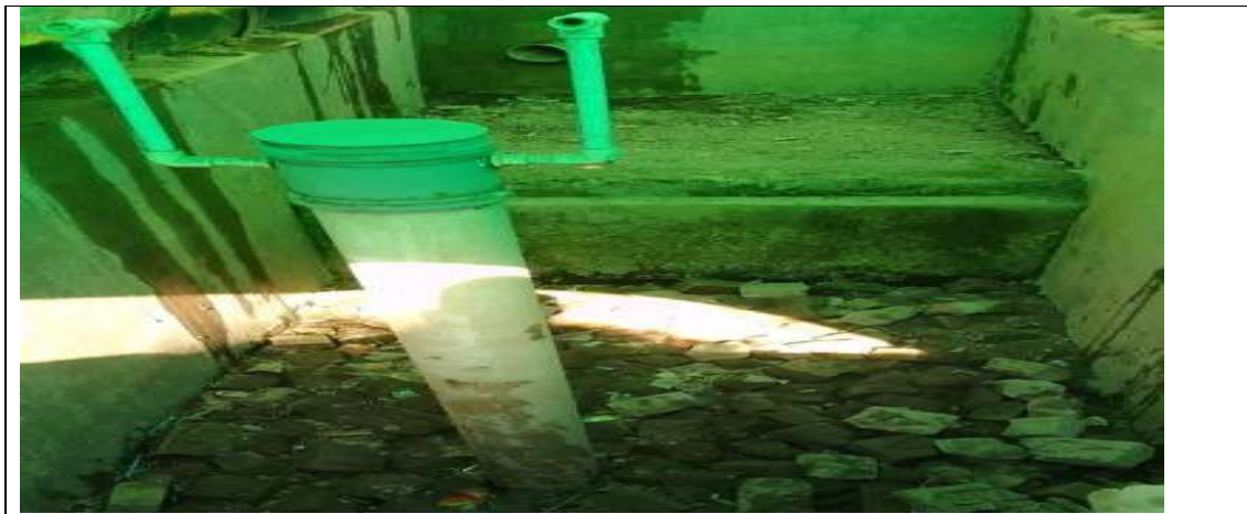
F9: Rainwater Harvesting System
